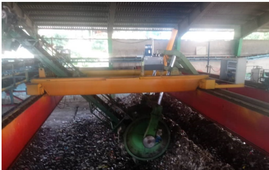
Figure 1. Composting windrows inside the roofed fermentation hall of the CPBM
